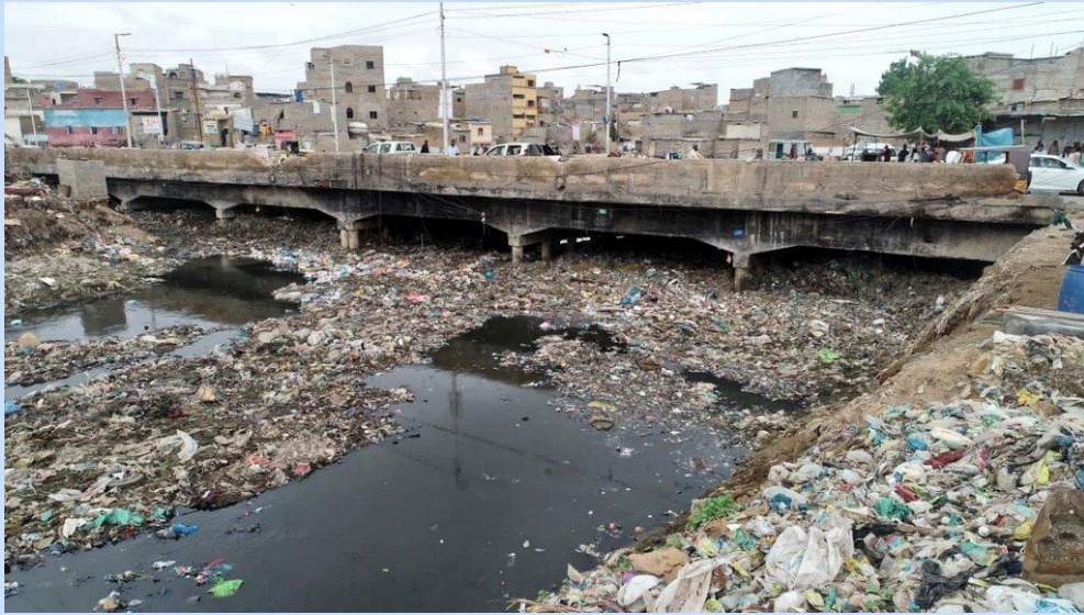
Nala choked with garbage
