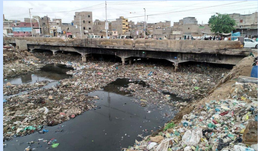
Nala choked with garbage
